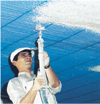
KaRo-Cooling Ceiling with katubes 1991 in a bank in Geneva
